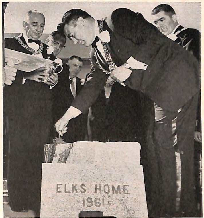
RENO, Nevada, Lodge's E.R. Albert Solari applies mortar in the cornerstone laying for the lodge's new home. Others include Est. Loyal Knight Don Rose, Past Grand Exalted Ruler H. R. Wisely, background, and Chaplain Louis Capurro, far right.
