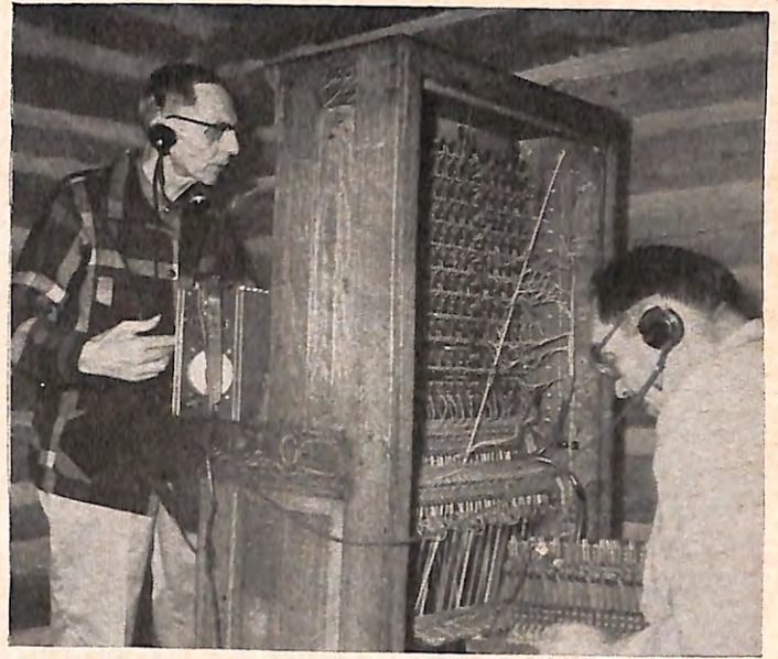
NORTH DAKOTA. Chester Cooch, a retired telephone man from Jamestown, left, and Charles Miner of Bismarck test the switchboard they helped to install at Camp Grassick, the camp for crippled children which is owned by the North Dakota State Elks Assn.
