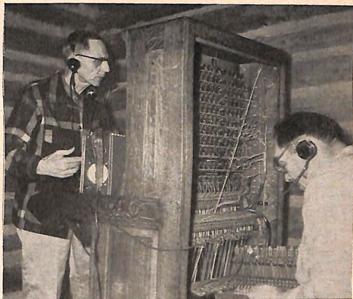
NORTH DAKOTA. Chester Cooch, a retired telephone man from Jamestown, left, and Charles Miner of Bismarck test the switchboard they helped to install at Camp Grassick, the camp for crippled children which is owned by the North Dakota State Elks Assn.
