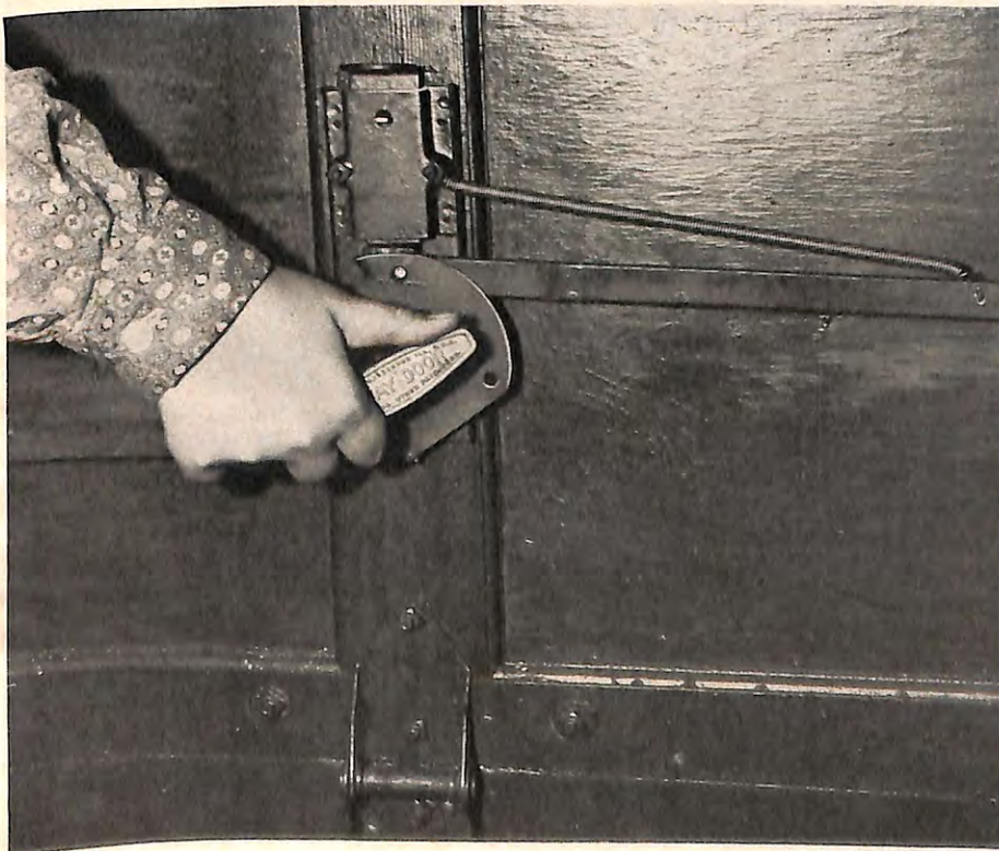
A broken latch spring is easily replaced by a screen-door spring. Hook at least two turns of it into a hole in a latch bar and the same over a bolt in the housing. Make sure both ends are securely engaged.
