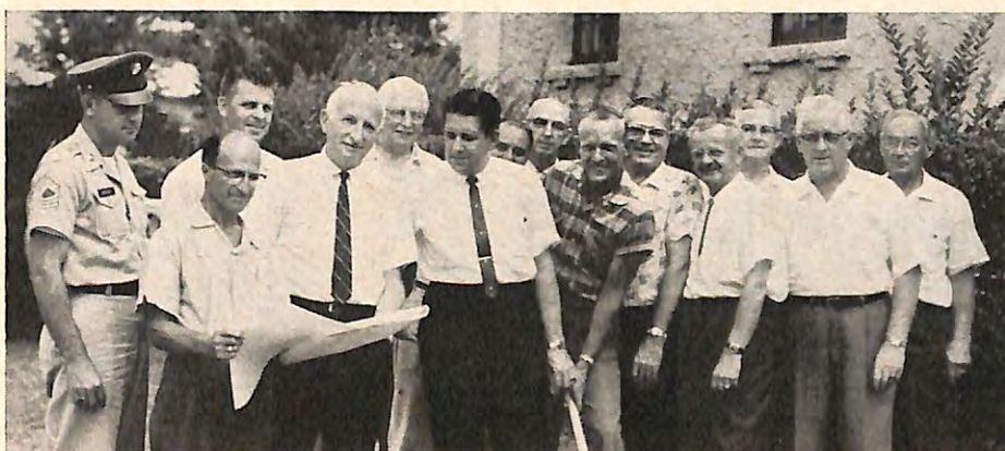
DeLAND, Florida, Lodge's Exalted Ruler Charles O. Benton, Jr., center, turned the first shovelful of earth for the new addition to the lodge's headquarters. Others pictured are, left to right, Morton Marsh, George Napoli who is the construction representative for the project, Bill Kauffman, Stanley Hodes, Glenn Wheeler, Clyde Lankford, Frank Vetere, Paul Thomas, Carl Minz, Past Exalted Ruler Frank Kauffman, Ed Taylor, Mike Roach and Past Exalted Ruler George Hindery. This project, made necessary by the increase in membership and the wider range of activities in which these Elks are interested, will give an additional 2,000 square feet to the lodge's present facilities. Construction on this addition is now well under way and the Elks are preparing for their opening celebration.
