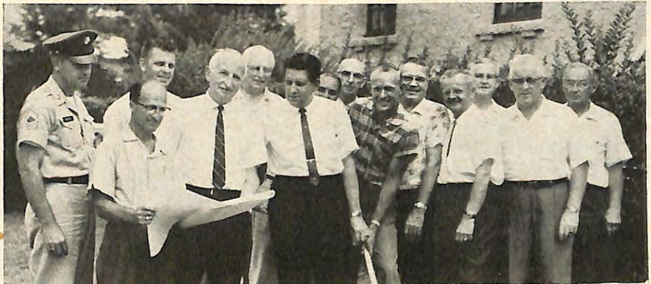
DeLAND, Florida, Lodge's Exalted Ruler Charles O. Benton, Jr., center, turned the first shovelful of earth for the new addition to the lodge's headquarters. Others pictured are, left to right, Morton Marsh, George Napoli who is the construction representative for the project, Bill Kauffman, Stanley Hodes, Glenn Wheeler, Clyde Lankford, Frank Vetere, Paul Thomas, Carl Minz, Past Exalted Ruler Frank Kauffman, Ed Taylor, Mike Roach and Past Exalted Ruler George Hindery. This project, made necessary by the increase in membership and the wider range of activities in which these Elks are interested, will give an additional 2,000 square feet to the lodge's present facilities. Construction on this addition is now well under way and the Elks are preparing for their opening celebration.
