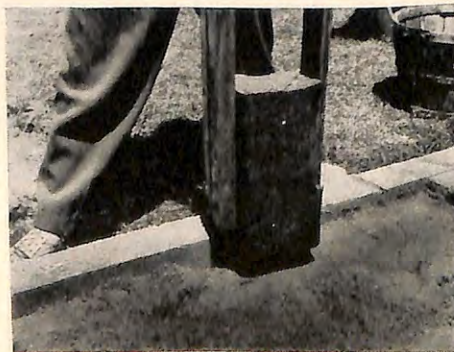
Tamping the sand base insures a firm bed and reduces shifting of paving units.
