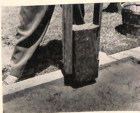
Tamping the sand base insures a firm bed and reduces shifting of paving units.
