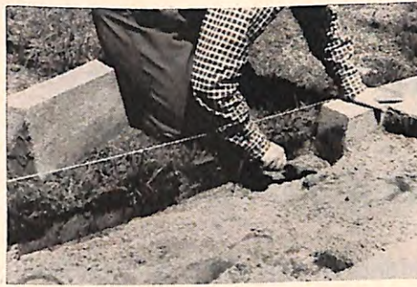
Rectangular flagstones are easy to lay. Remove sand or tamp more under them as needed to align the joints. Block border retains sand bed above level of lawn here.
