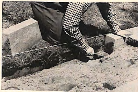
Rectangular flagstones are easy to lay. Remove sand or tamp more under them as needed to align the joints. Block border retains sand bed above level of lawn here.
