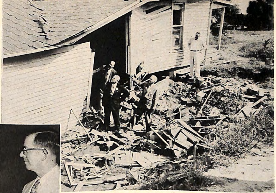
Above: Mr. Davis and Past Grand Exalted Ruler Henry C. Warner, with D.D. W. C. Hunsinger and E.R. Dick Pucka of Lawrence, Kans., inspect flood damage.
