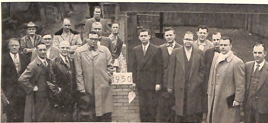
Exalted Ruler William J. Braddock, with fellow officers and the lodge Trustees, who are also members of the Building Committee, lays the cornerstone for the new home of Warsaw, Ind., Lodge.
