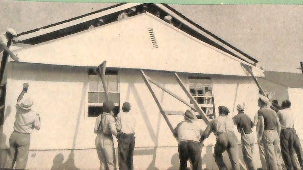
A prefabricated demountable house which can be taken down, moved and erected again in less than a day.
