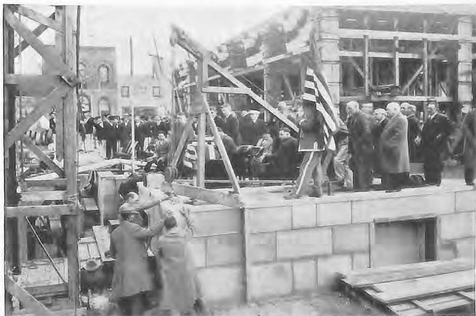
The laying of the cornerstone of the new Federal Court Building in Prescott, Ariz., at which the officers of Lodge No. 330 in that city presided
